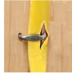
Insulation in cables can be severed if a staple is misapplied.
