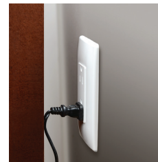
Furniture pushed against the plug of an appliance cord can stress conductors and damage insulation.
